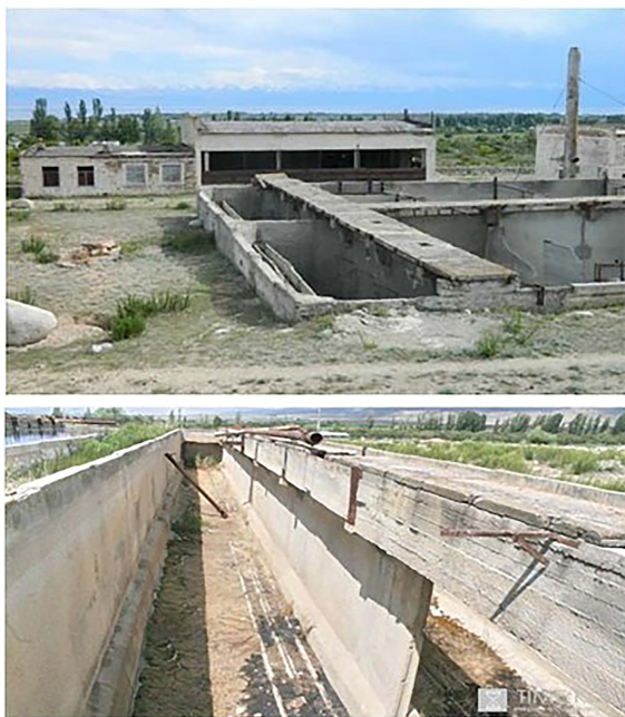
Figure 1. Wastewater treatment facilities of the "Vodokanal" enterprise in Cholpon-Ata city
